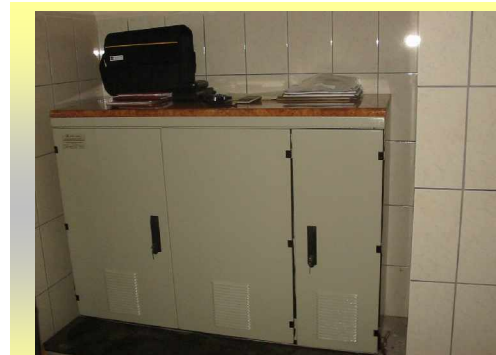
Electric switch box for instrument
