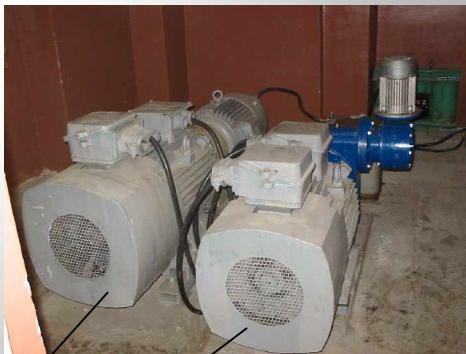
1 2 Groups of machines from the transformer
