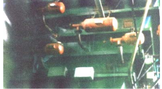
COAL Metallic Bunker THERMOELECTRIC POWER BRASOV-ROMANIA
