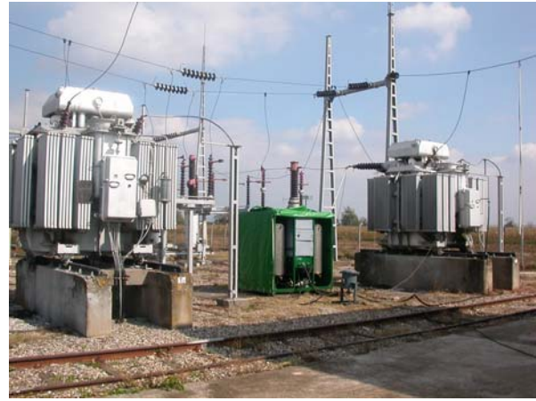
Fig. 3 VIMAP R2000 installation in operation
